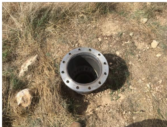
Borehole with flange
